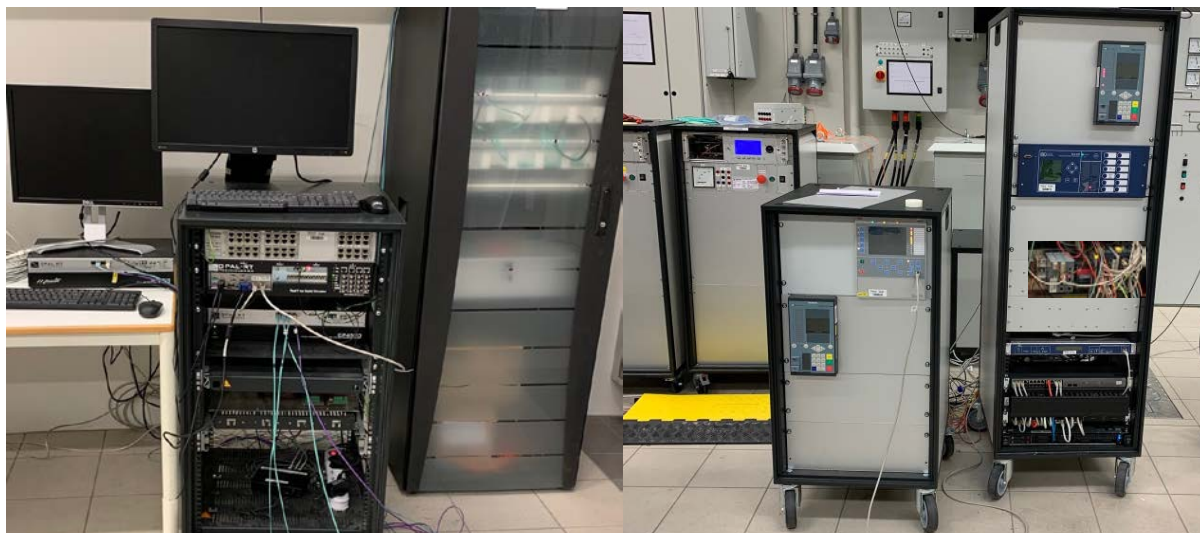
Figure 11 NSGL flexible digital substation equipment. (Left) DRTS from OPAL-RT and optic fibre rack. (Right) Multiple vendor MUs, IEDs, GPS clock and communication switches.
